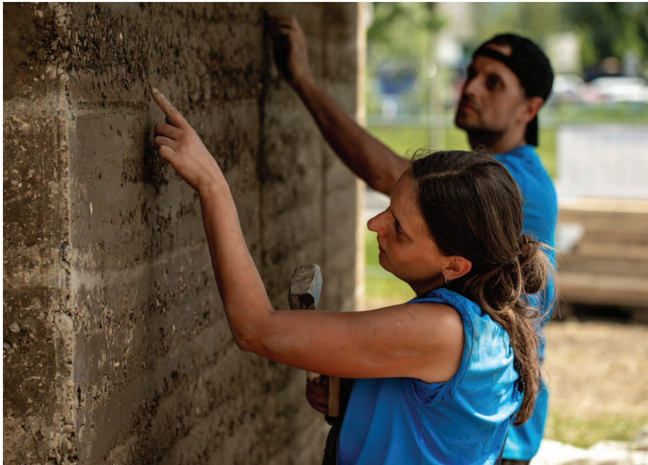
Learning on a real scale. Retouching a rammed earth wall during a workshop with Lehm-Ton-Erde Baukunst GmbH in Wolfurt, Austria (2022).
