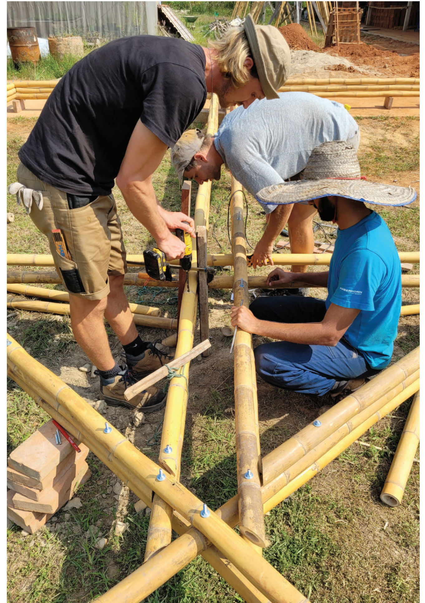
Exploring local bamboo as a building material. Hands-on experience in Thailand, building a sustainable agriculture centre for the NGO Baan Doi.
