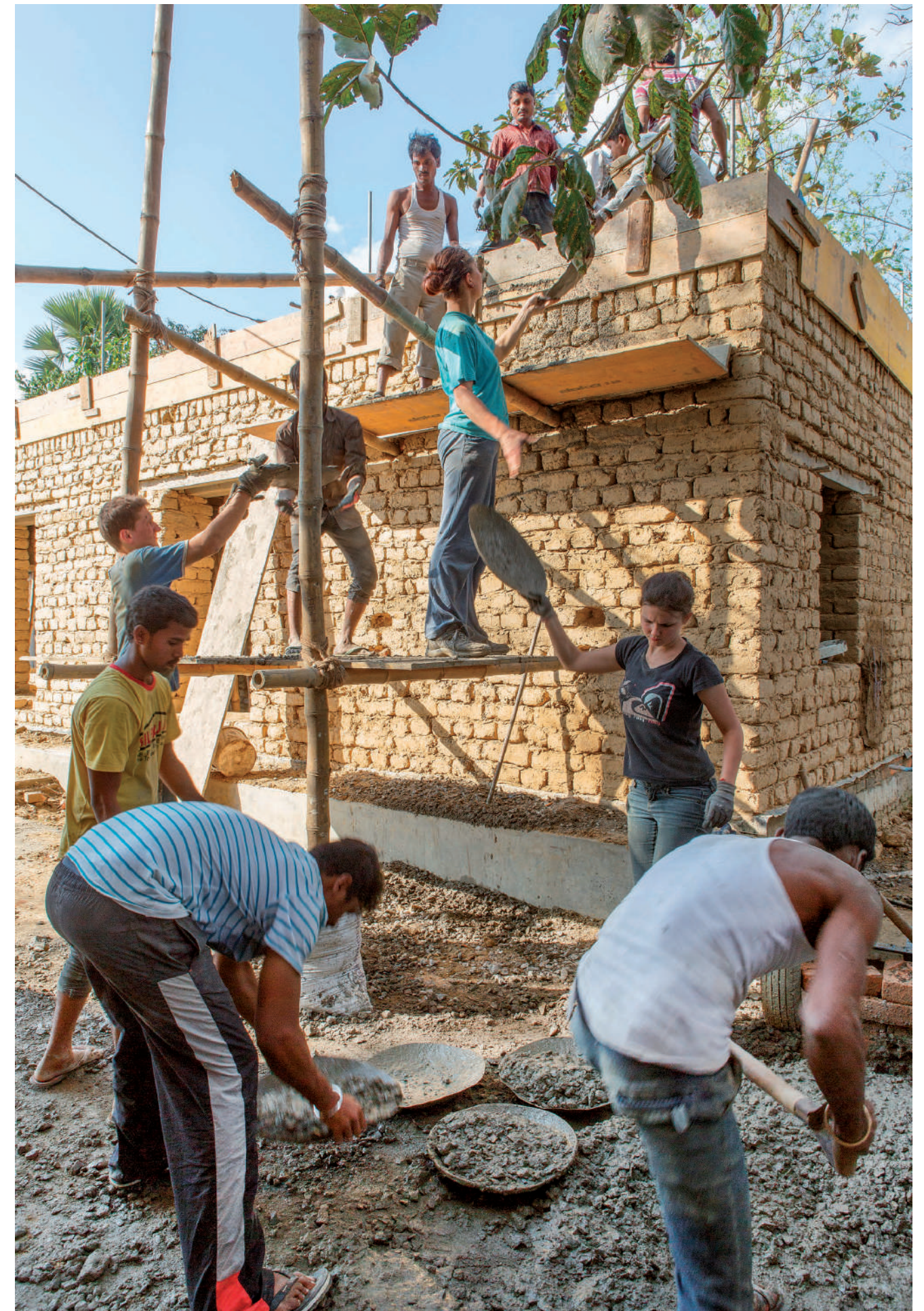
Learning together: hands-on experience for students and craftsmen on the construction site of teachers' housing in Sunderpur, India (2012-2015). Credits: Stefanie Hueber
